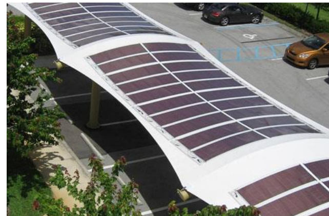
Flexible PV modules on parking lot canopy: Konarka Technologies, Inc.
